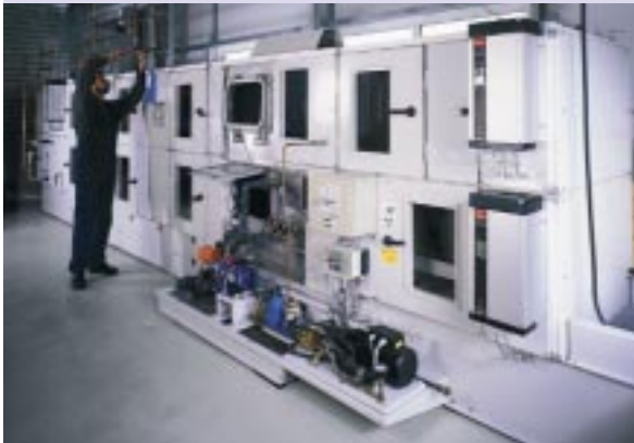
Fig. 1: The air-handling unit is the core of the test stand for desiccant cooling systems.
