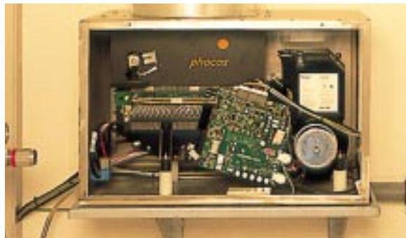
Fig. 3: A hydrogen-fuelled, polymer-electrolyte-membrane (PEM) fuel cell with a power rating of 1.2 kW is being operated at the "Rappenecker Hof". The PEM fuel cell (its stacks can be seen in the background) requires pure hydrogen and atmospheric oxygen for operation.
