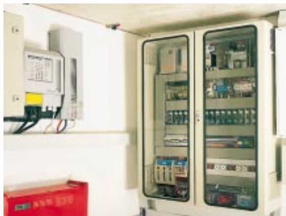
Fig. 4: Control panels for the entire household power supply.
