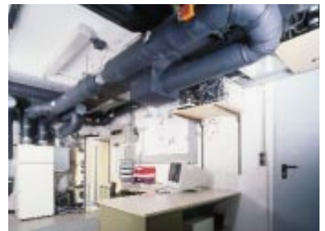
Fig. 3: Automated test stand for simultaneous measurement of two ventilation pumps with integrated exhaust-air heat pumps.
