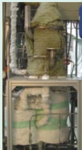
Fig. 2: Complete view of the thermally insulated, natural gas reformer. The reformer reactor itself is in the lower part of the system, the CO shift and methanisation reactors are located above it.
