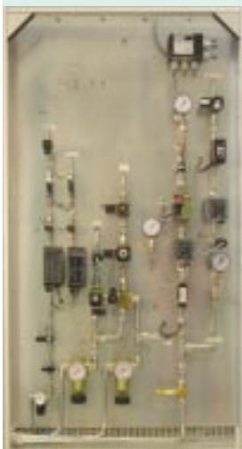
Fig. 1: View of part of the newly developed natural gas reformer. The components for dispensing the educts and the burner supply can be seen. Automatic burner control (upper right), controls for the feed (centre), feed lines (below).
