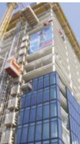
Fig. 2: The "Messeturm" (trade fair tower) in Basel, Switzerland. In the highest building in Switzerland, the exhaust air is removed from the rooms via the intermediate space in the facade. This air flows past the sun-shading units, cooling them and the intermediate space. The photo shows the installation of the facade elements.
