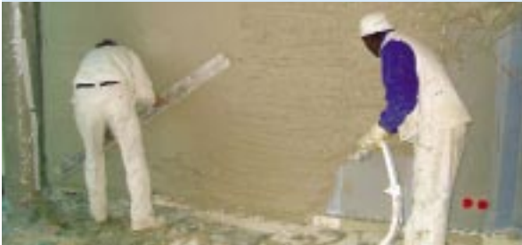
Fig. 1: Application of the PCM plaster in the new premises of the badenova utility in Offenburg. The material can be handled on the building site in exactly the same way as conventional plaster.
